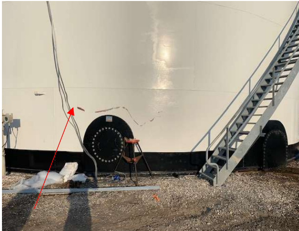
Scratches to tank 66
