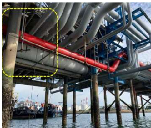
Approximate location where the deceased was working and location of scaffolding which fell.
